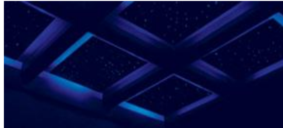
Accent lighting pre-installed on top of the perimeter
